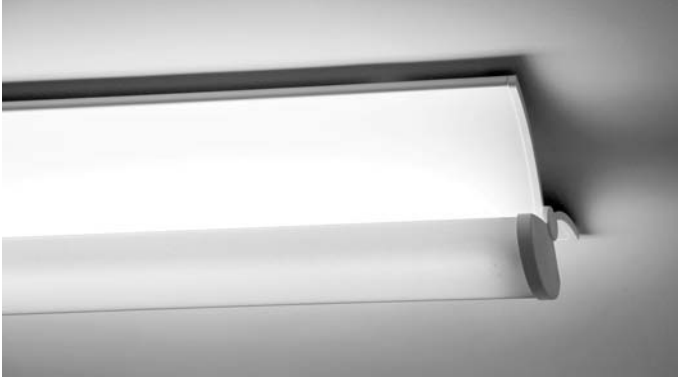
FIGURE 12.7 A view of a ceiling-mounted 'soft-light' luminaire.
