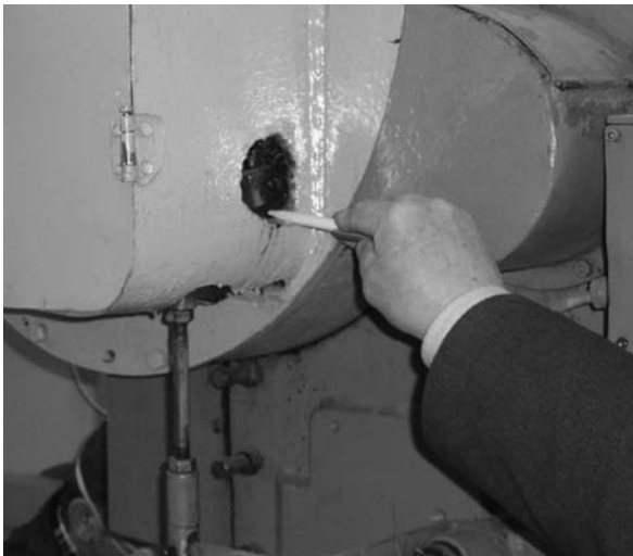
FIGURE 27.5 Requirements for safety distances are not satisfied.
