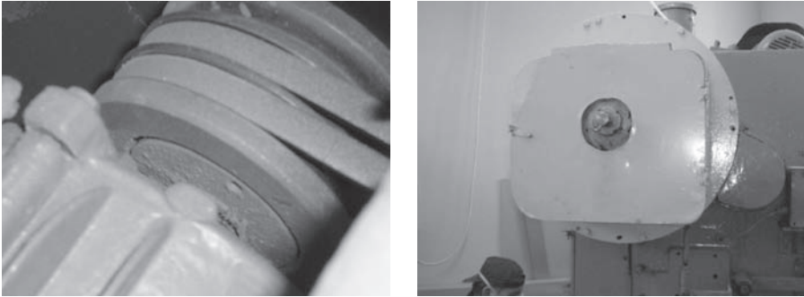
FIGURE 27.4 Lack of protection against rotating parts.
